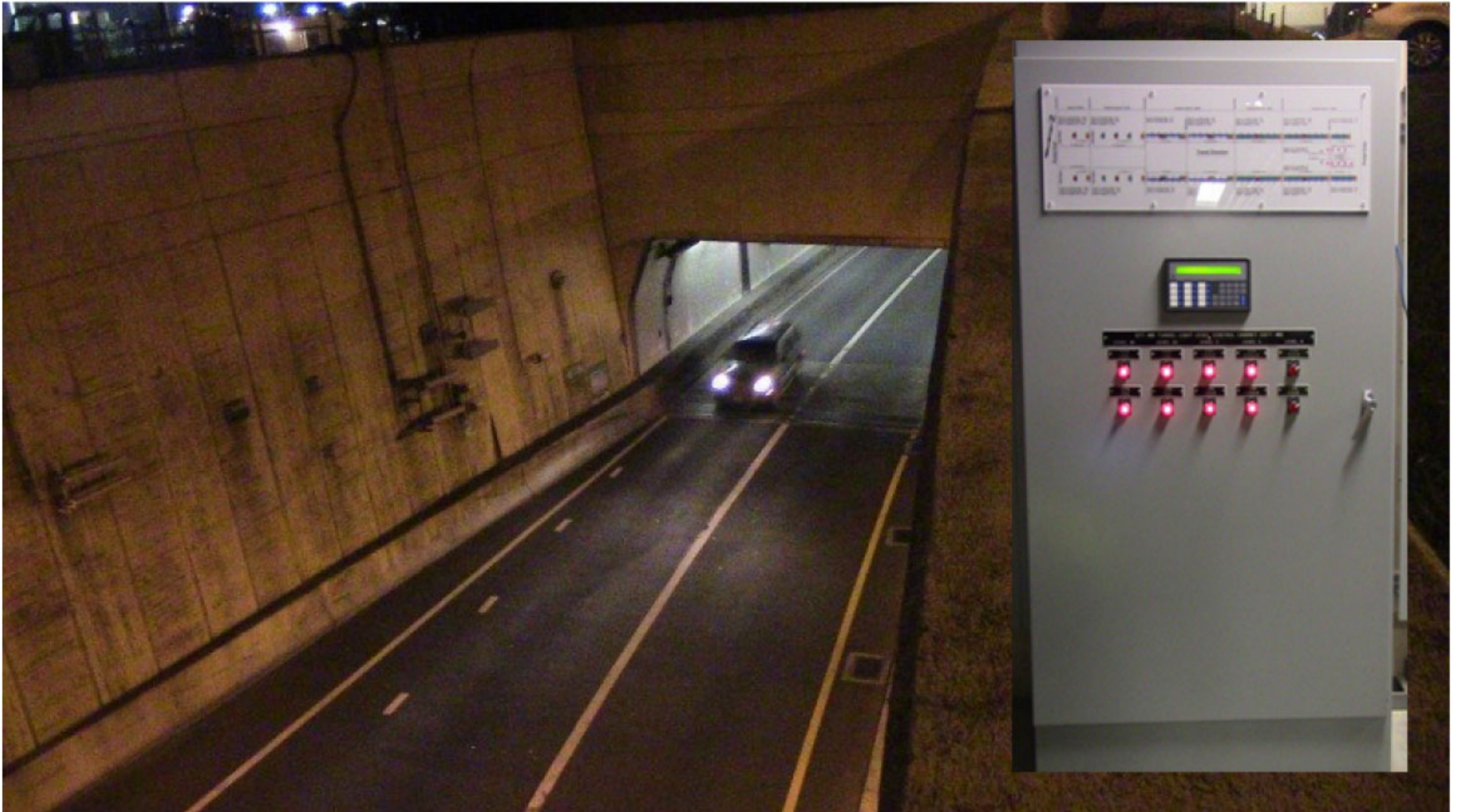
Portsmouth Downtown Tunnel | Tunnel Lighting Control System
